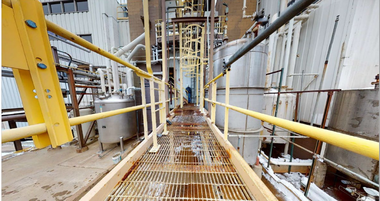
This photo shows CordenPharma's tank farm prior to the installation of new tanks and piping completed for the CordenPharma Project.
