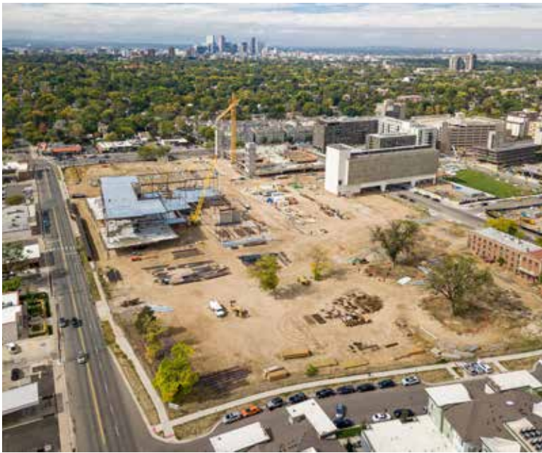
Southeast aerial view of the Commercial Area site. Preparations underway to set the final jumbo beams, 286,677lbs in total. This would complete the framework for the off-set second story of the movie theater. Photo by Two24media.
