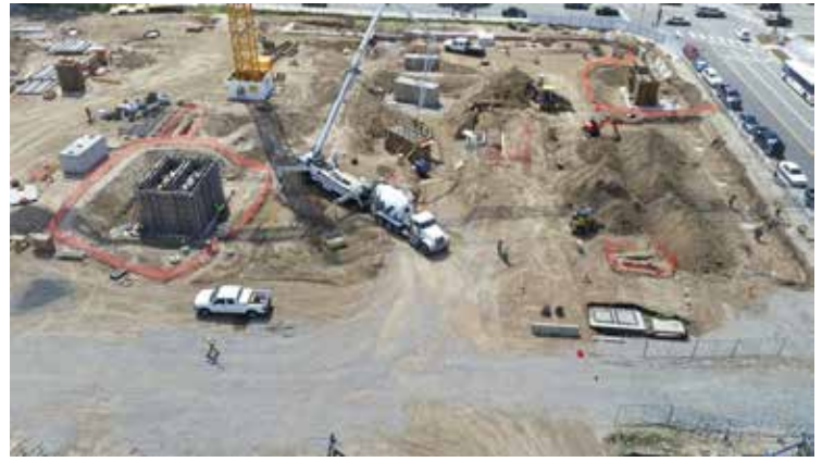
Turning a corner, Kiewit completes the last of four pier caps to bridge across existing deep foundations left behind from the previous building. The last two pier caps were 21ft x 7ft x 9ft and each spanned across two 6ft x 25ft drill piers, in total adding over 200 cubic yards of concrete to the project. Photo by Sensera Systems.
