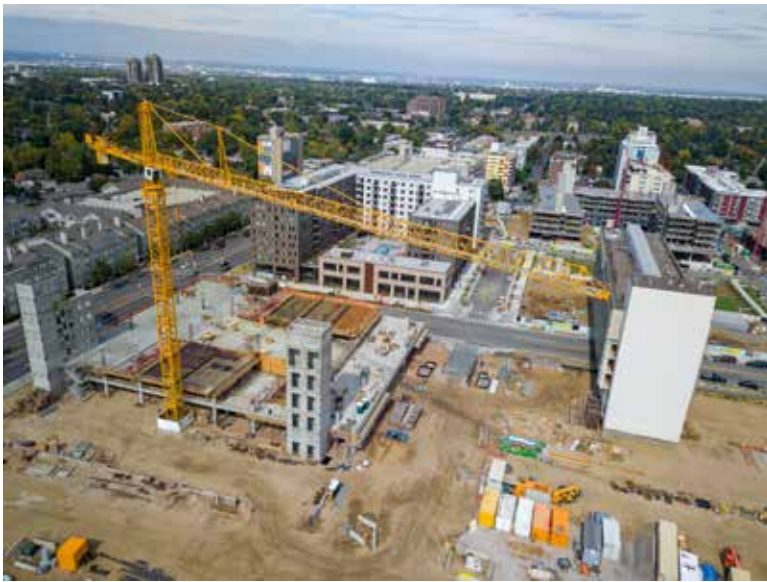
Birds-eye view of the Block 4 construction. Ahead of schedule, the north and south deck of Level 3 are being prepped for a simultaneous pour. In total, there would be twenty four deck sections and over 8,000 cubic yards of concrete placed. Photo by Two24media.
