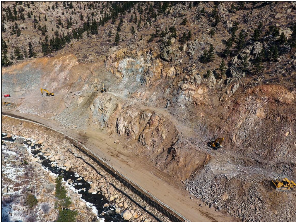
Crews blasted and hauled more than 380,000 cubic yards of rock in making US 34 more resilient.
