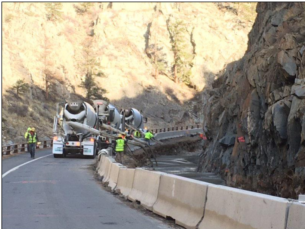
In the most narrow sections of the canyon, crews mixed dense bedrock material with concrete to create a 15-foot wide section of roadway that is more resilient to the eroding effects of water.
