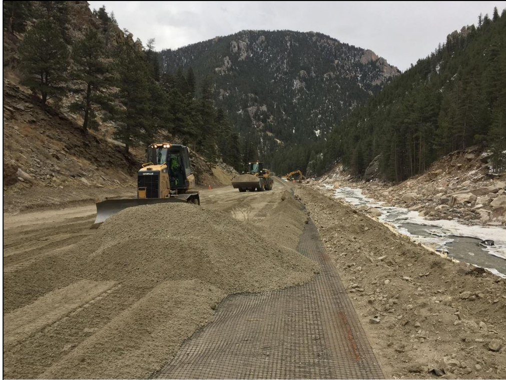
After installing grouted riprap beneath US 34 to help it better withstand the eroding effects of water, crews grade the sub-base course prior to putting down the base course and then paving the roadway surface.
