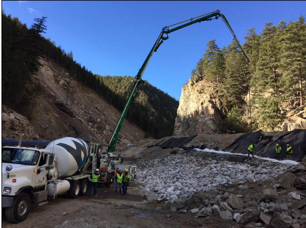
To help make US 34 more resilient to flood damage, crews put in several layers of riprap beneath a section of the highway and then grouted the void areas between the large rocks.
