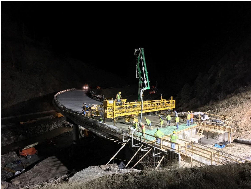
To minimize the impact on Big Thompson Canyon residents trying to get into and out of the canyon, Kiewit crews worked overnight to pour the deck for the new horseshoe curve bridge structures.
