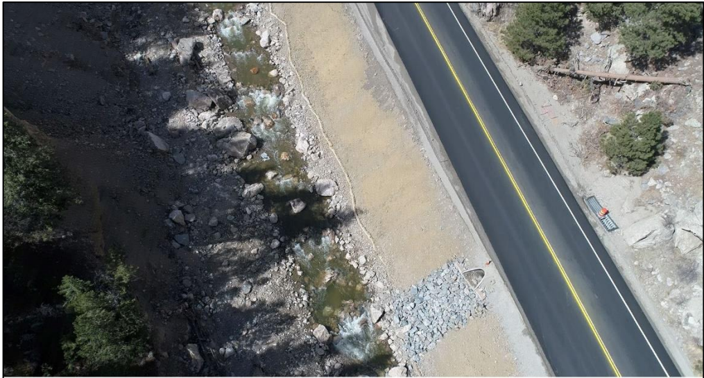
New drainage structures with riprap armoring will help protect US 34 from future damage.
