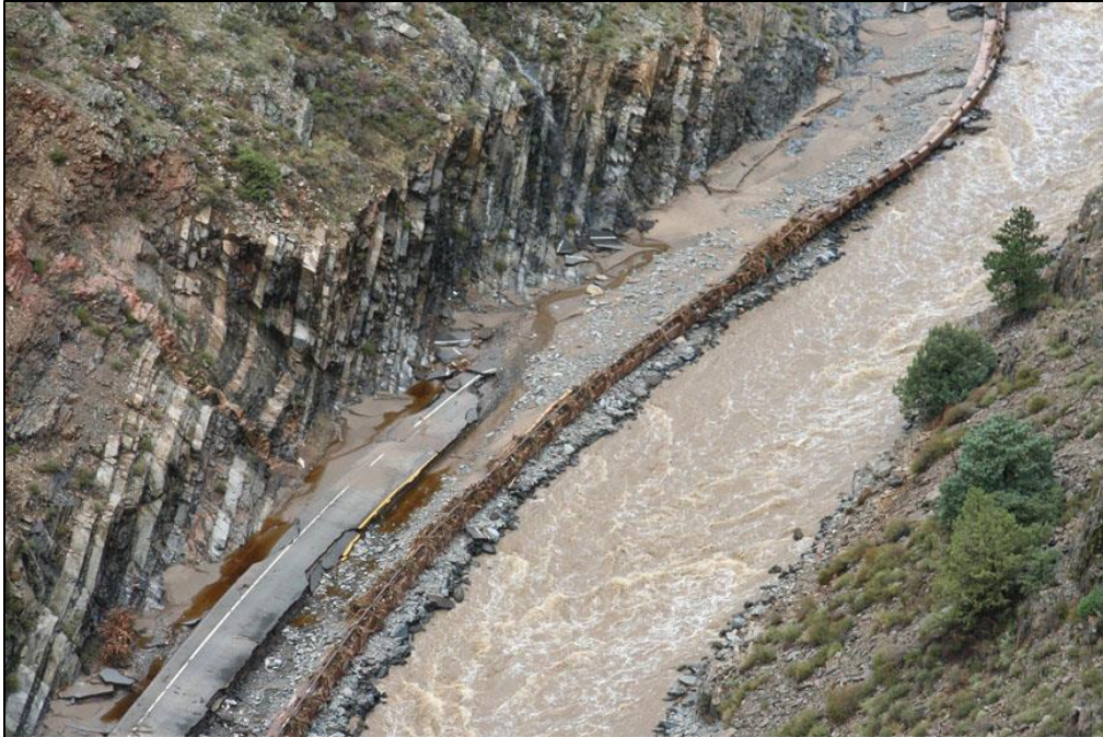
Whole sections of US 34 between Loveland and Estes Park washed away in September 2013, trapping residents inside the Big Thompson Canyon and making it difficult for emergency crews to reach them.
