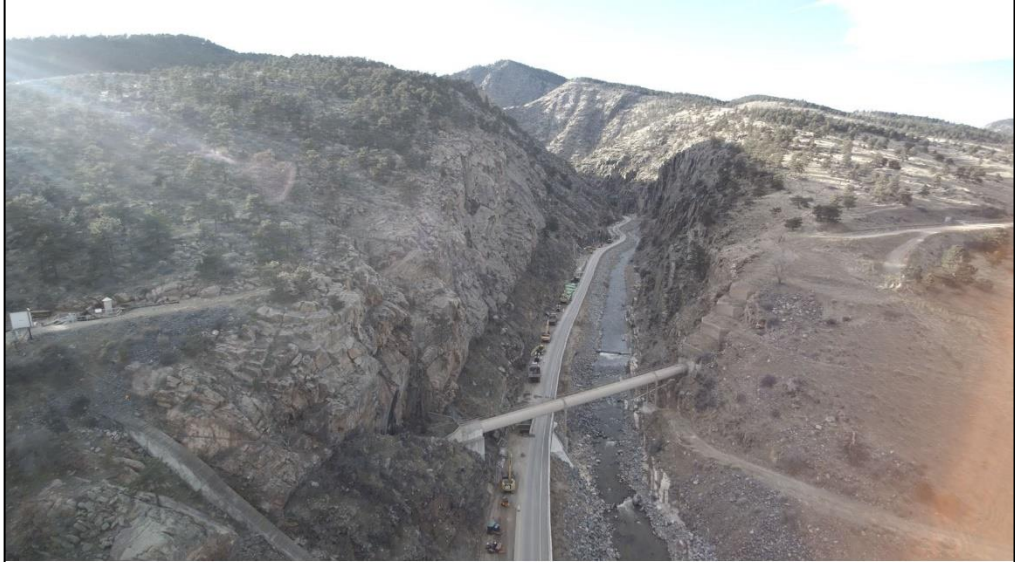
Soil cement mixing operations were effective in the tight right-of-way conditions dubbed "the narrows."
