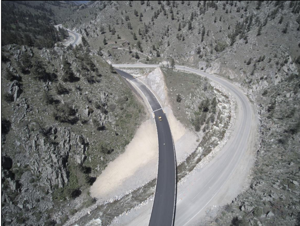
To better protect US 34 from future flood damage, Kiewit Infrastructure realigned the roadway through a rock cut and elevated the highway above the Big Thompson River through the heart of the canyon.
