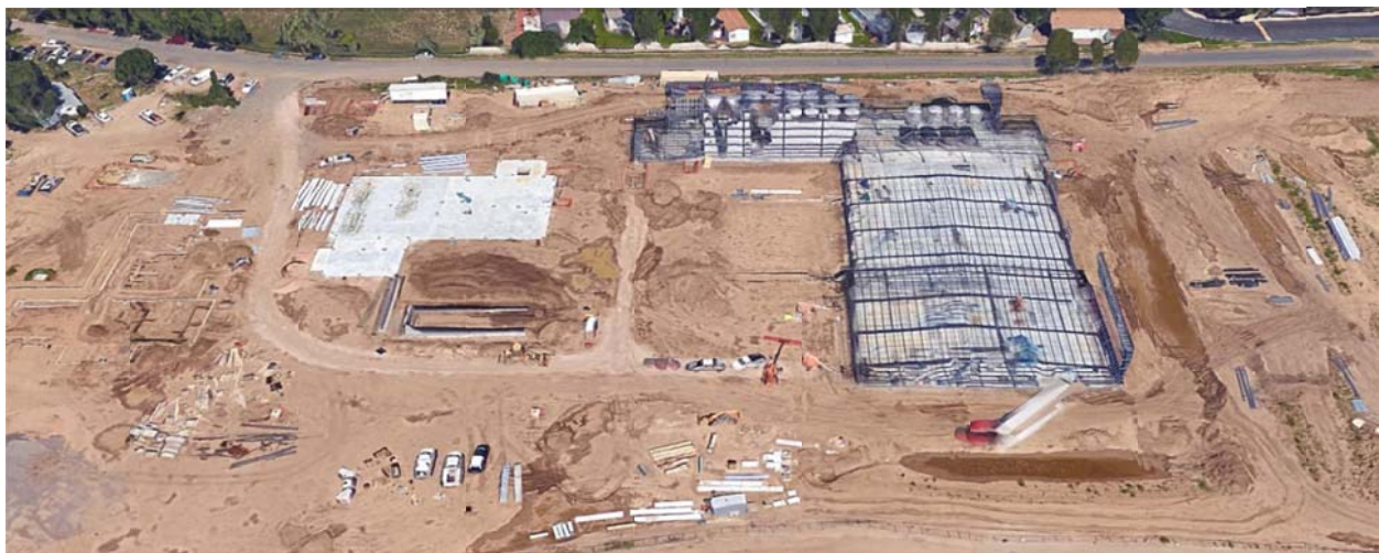
This Google Earth view shows the site on a typical day during its wet construction season.
