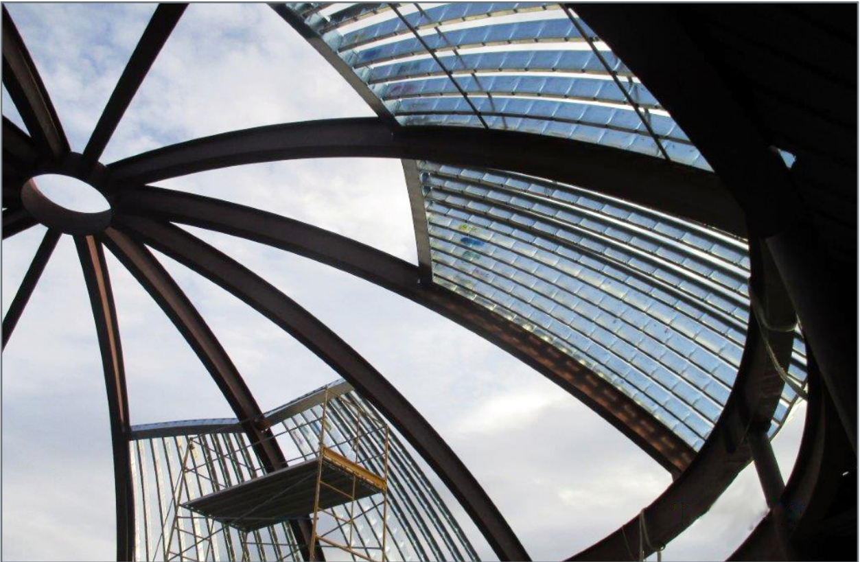
Four structural steel elements forming the basis of the dome were assembled and placed in one crane hoist. Installation required diligent safety planning and performance, and was aided by 3D laser scans imported into the BIM model to ensure fabrication and placement of in-fill framing.
